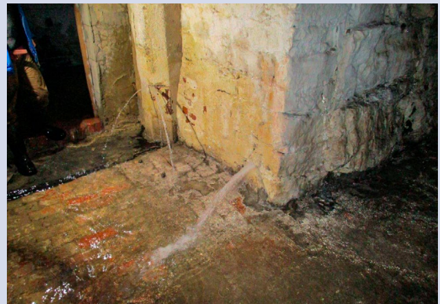
Water penetrating the cellar areas.
