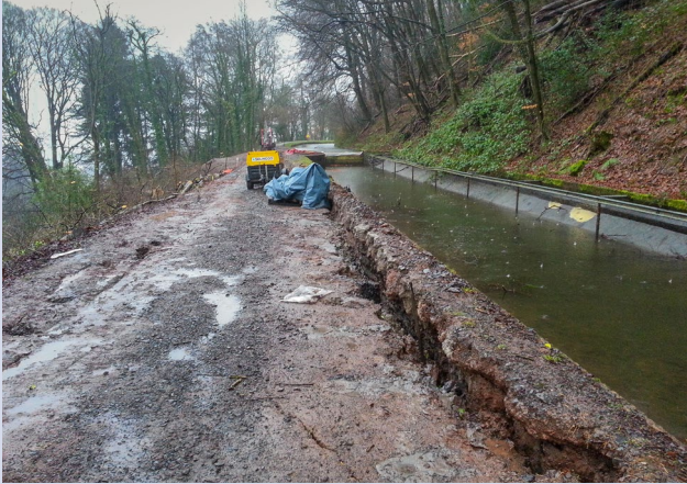
Grounding slumping away from the concrete lining of the canal near Tod's Bridge.
