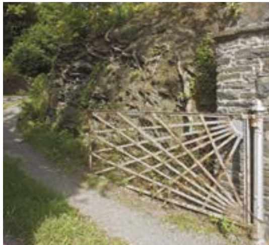
Ornament was important for suburban houses — both for the buildings themselves and for their boundaries. Ironwork detail was probably made locally (Crown Copyright: RCAHMW).
